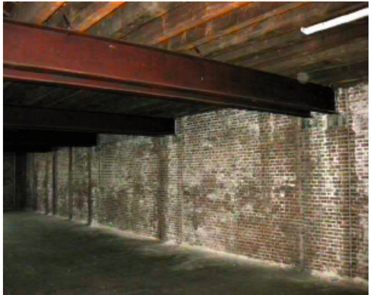
Image 4: 4th floor ceiling
